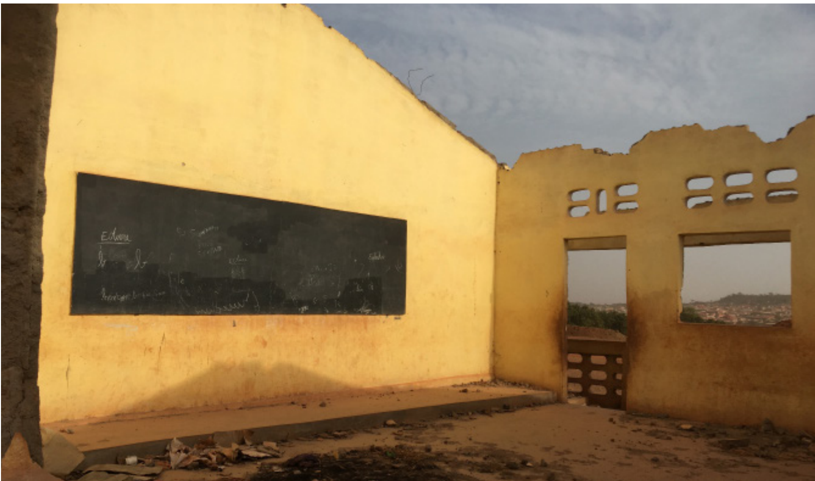
Residents had little time to prepare for the evictions. Most homes and buildings have already been demolished, but the remnants of this school still stand. (Credit: Inclusive Development International)
